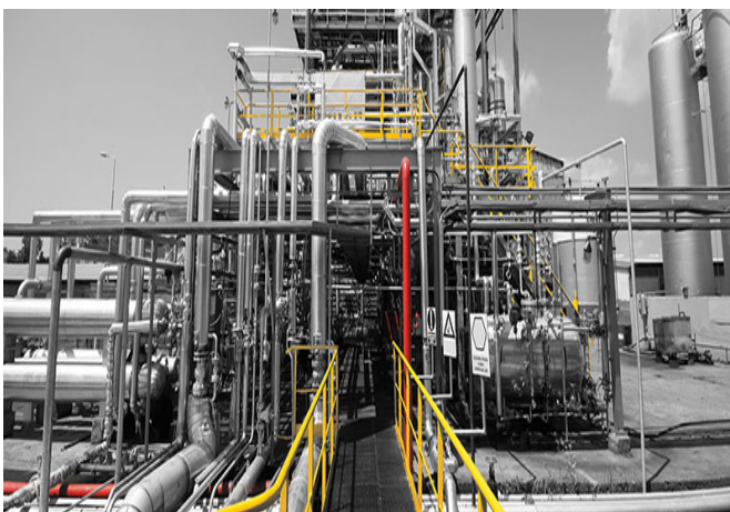
Gas & Oil Factories, Hot Pipe & Floor Area
